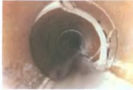
Fig 4.7 Root intrusion within a sewer pipe.
