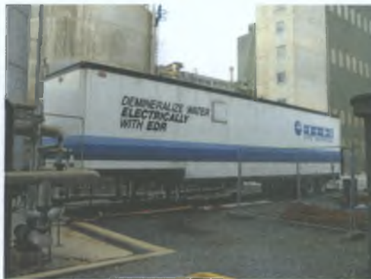
Plate 1: Electrodialysis Plant used at IFI, Arklow
